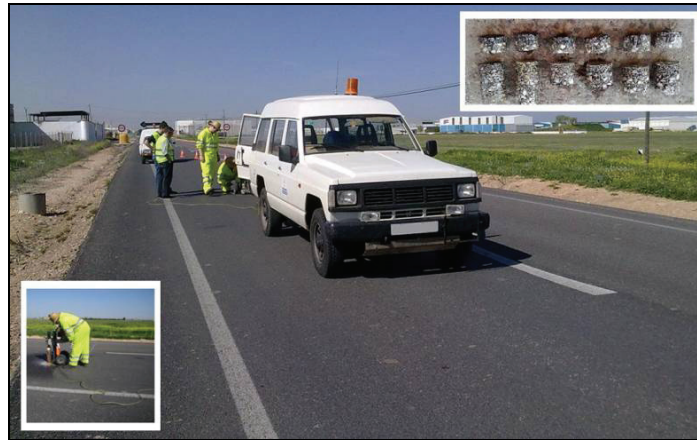
Fig. 2. Detail of the core sample extraction, asphalt pavement and core samples extracted
